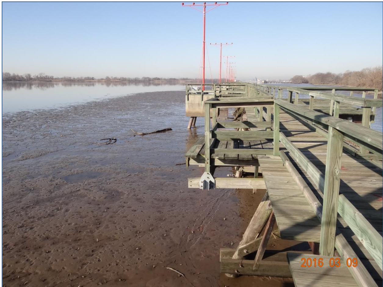
Photo 1: View from the east end of the existing 1,800-foot long timber walkway toward the western end showing the series of approach light standards attached to concrete dolphins, each 100 feet apart. Photo was taken at low tide which exposes a large expanse of tidal marsh (tips of the spatterdock plants are visible at the numerous dots in the mud surface.)
