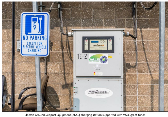
Electric Ground Support Equipment (eGSE) charging station supported with VALE grant funds
